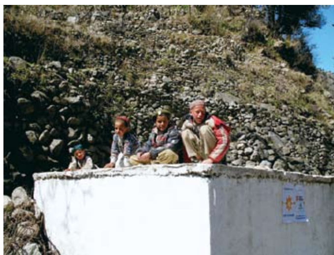
Reconstruction of water collection tank in remote Himalayan village after earthquake, Pakistan
